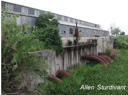
This 100-year-old water pumping plant in Cameron County was in need of modernizations to more efficiently conserve water.
