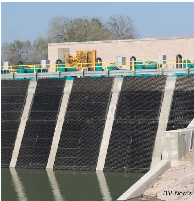
This new pumping plant is equipped with eight highly-efficient pumps, which consist of four different sizes that pump water at various rates.
